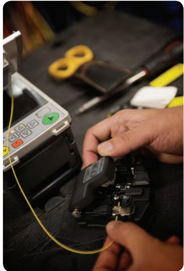
Fibre Field Termination
