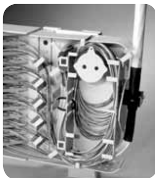
IFC Cables Loaded into FTB
